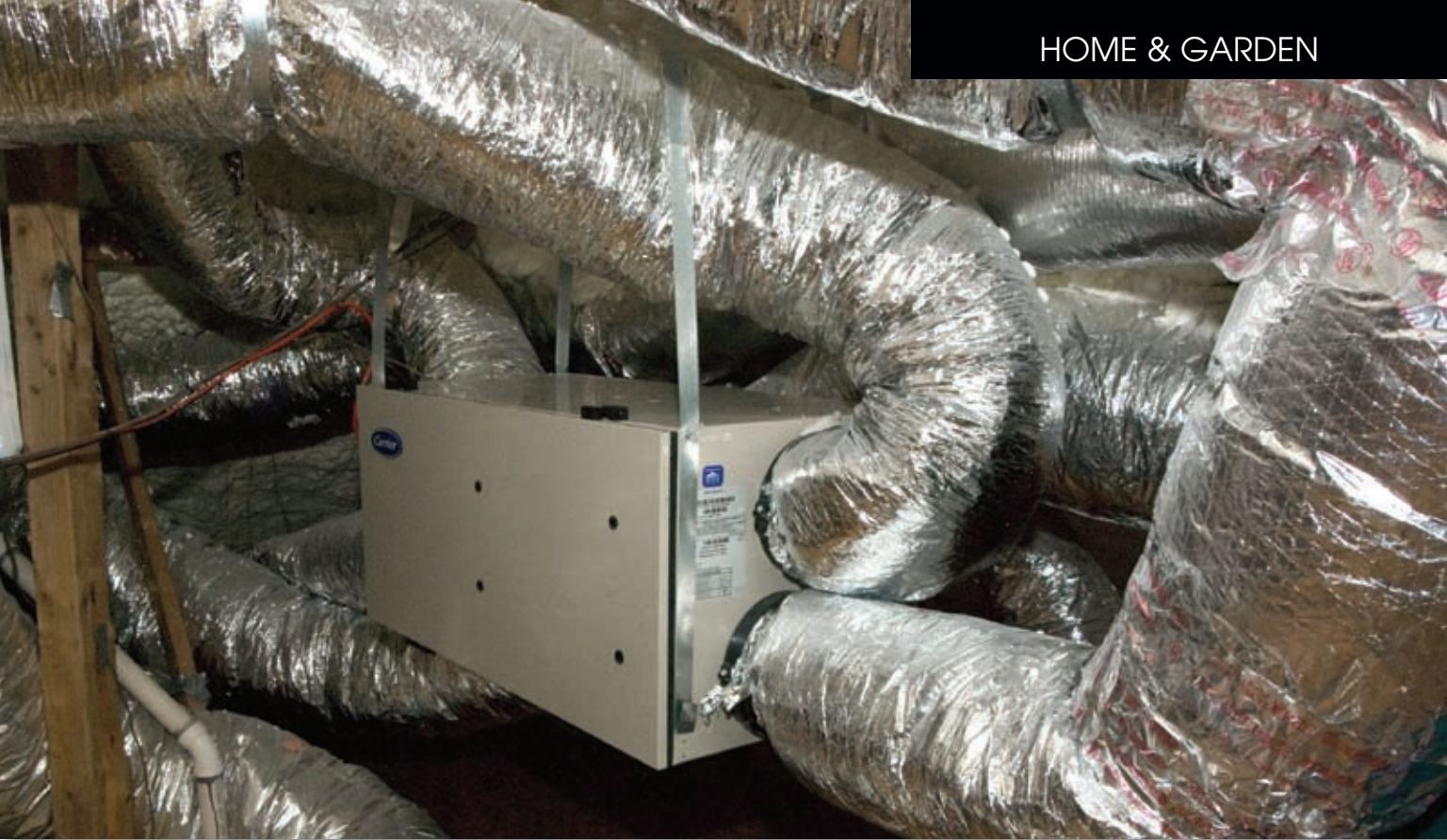
Typical home ductwork
